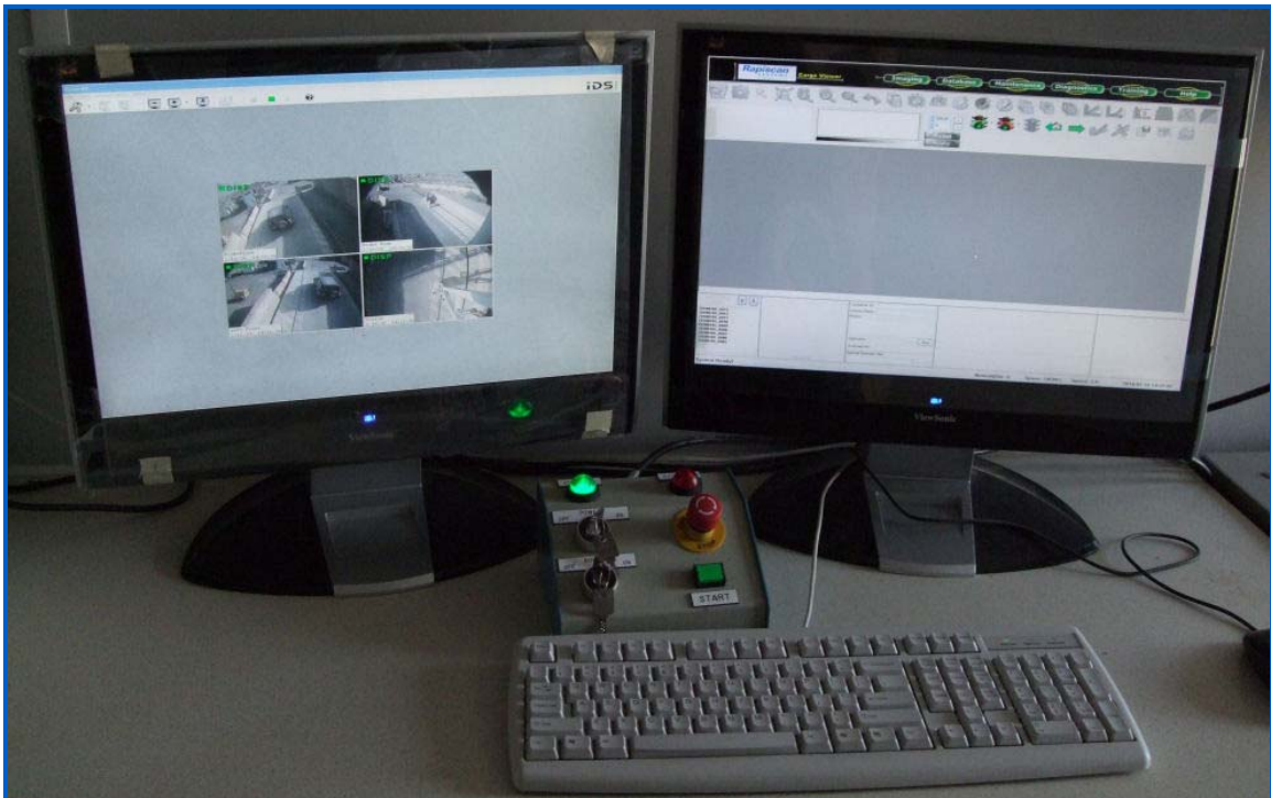
Figure 4: Operator Workstation Desktop Components
