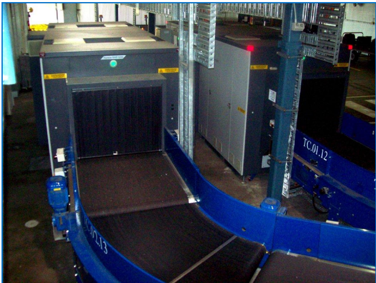
Figure 2: X-Ray Scanners "Inline" with an Airport BHS
